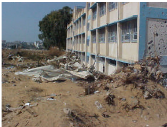
Photo 3: Jabalia Prep "A" Boys School, October 2004. The complete destruction of the southern boundary wall was caused by debris pushed onto the wall by IDF bulldozers.
