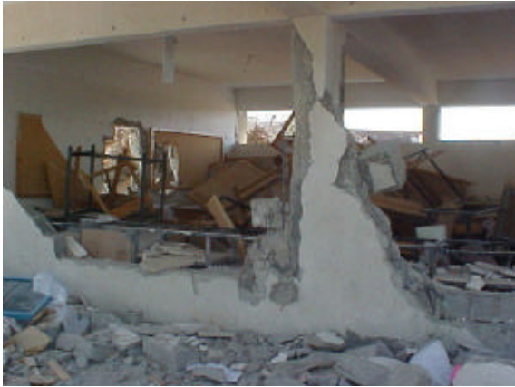
Photo 2: Jabalia Prep "A" Boys' School, hit by IDF tank shells, Oct 2004
